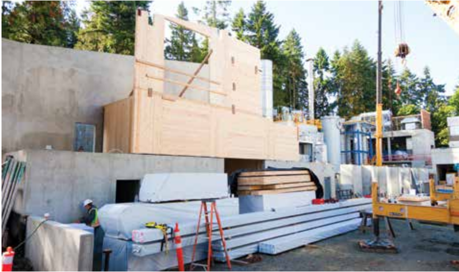
Once delivered to the construction site, wood should be stored and wrapped properly.
