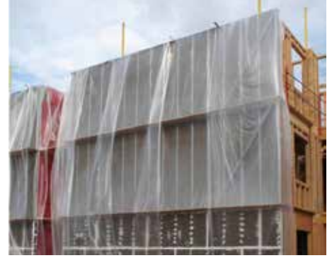
This photo shows how a multi-story wood building can be protected from the elements.
